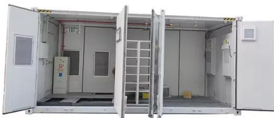
1075KW HH ESS
