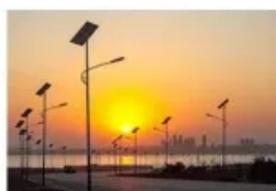
Solar Street Light
