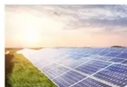
Energy Storage System
