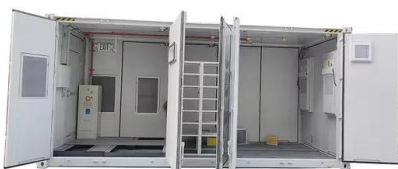
1075KW HH ESS
